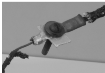
Fig. 5. Connection between copper cable and aluminium joint only minutes before the joint destruction
