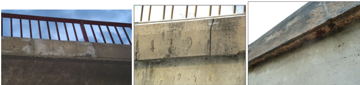
Fig. 2. Samples of steel corrosion and spalling of concrete on concrete cornices
