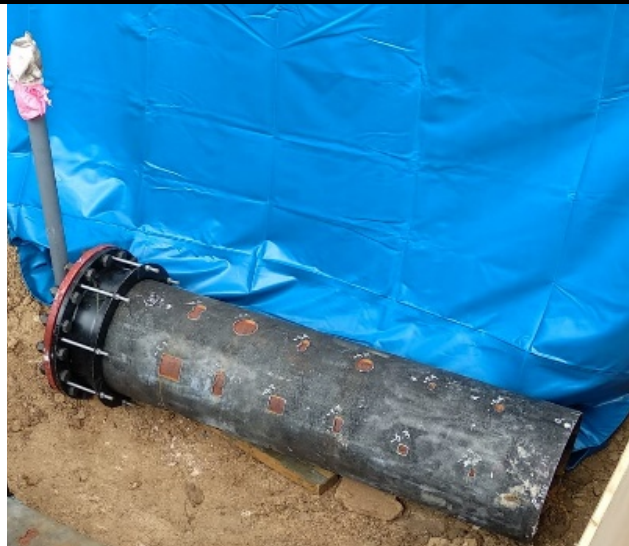
Fig. 1: Pipe sample with milled defects on the pipe exterior before buried attached with a flange connected to a riser pipe with shut off valve at the left of the pipe.
