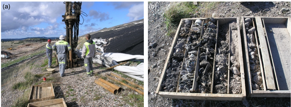
Fig. 4. Borehole B1: a) drilling of borehole; b) extracted material up to a depth of 6 m
