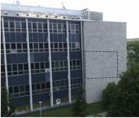
Fig. 1 Photo of the wall of the Vachon building inspected in article [3]. The area of interest is outlined by a black rectangle.
