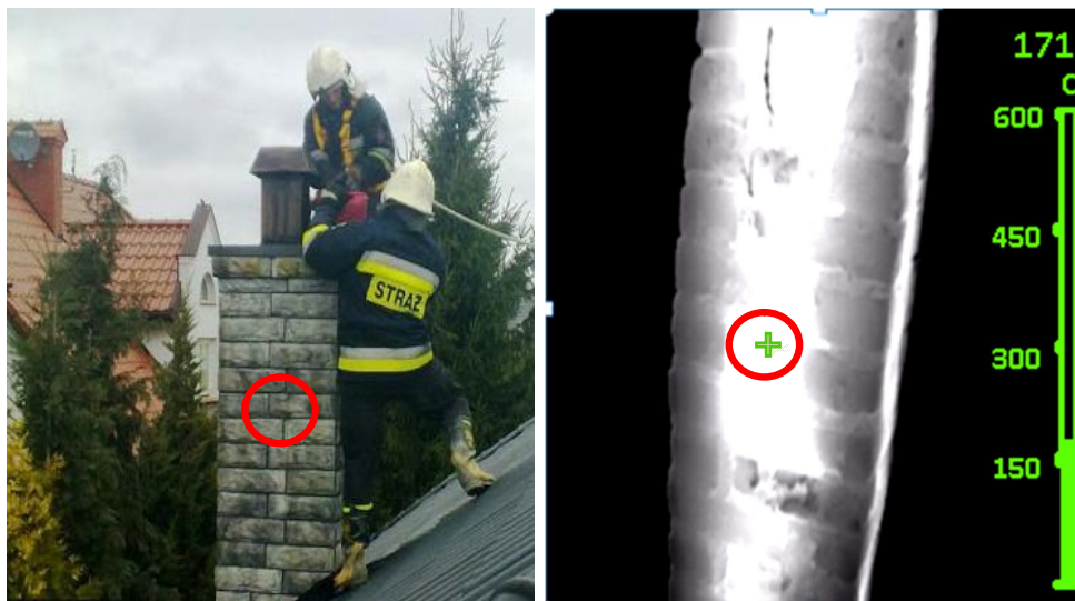
Fig. 4. A picture and a thermogram of a chimney. The temperature at the marked place was 171°C. Photo: Adrian Kwinciak
