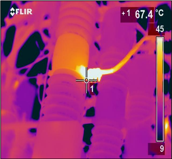
Hot-spot located on the breaker connections in Receiving Station
